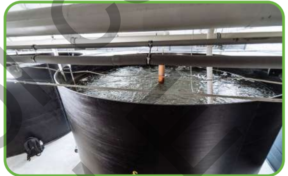
In tanks (indoor or outdoor)
